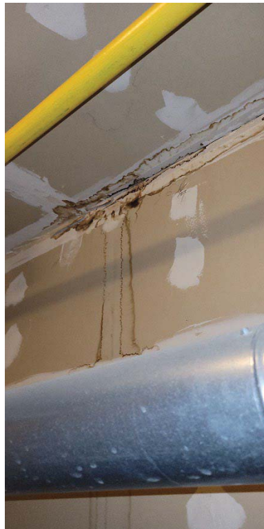
Photo 16: Leaks, ceiling of mechanical room
