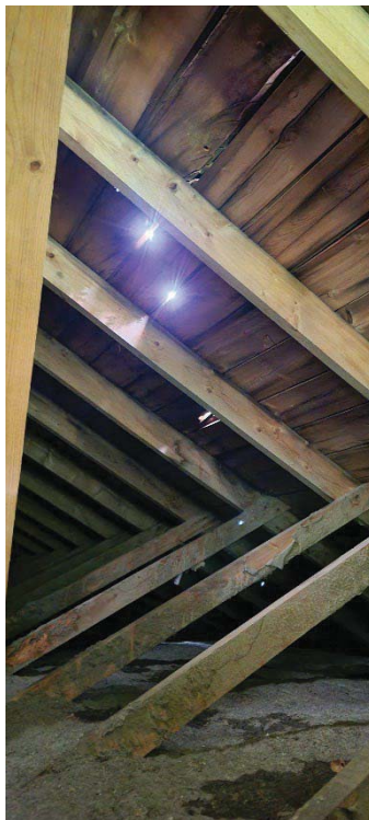
Photo 18: Daylight visible through attic above hall
